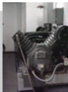
Air Compressor – Full Visible
