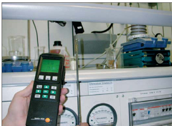
On-site testing of a laboratory exhaust fan with the testo 400
